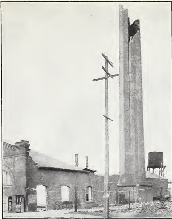
A. EARTHQUAKE DAMAGE TO BRICK STACK OF STAR SECTION, VALENCIA STREET POWER STATION, SAN FRANCISCO.
